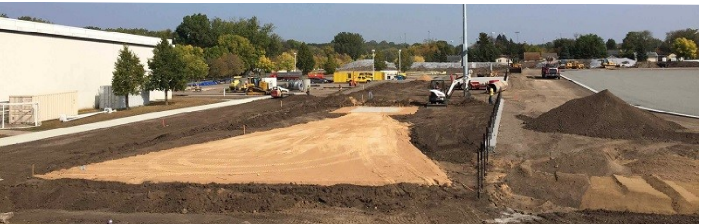
Images from top then left to right: Tennis courts mostly completed; excavation for stormwater management system with covered stockpiled urban fill visible at right; track and field area prepped for installation of shock pad and synthetic turf with LED field lighting in the background; shot put area under construction with the start of site fencing. (September 2020)
